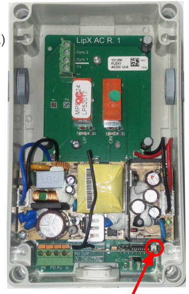
PROGRAM BUTTON (FLEX1-ACDC TRANSFORMER)
